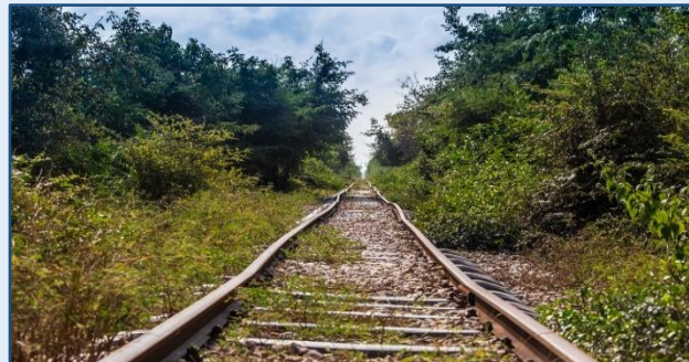
The Bent, Wrong Track
